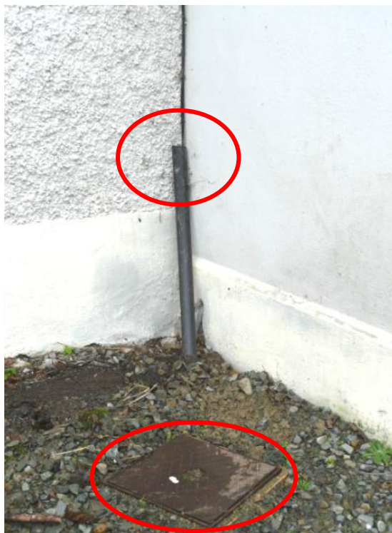
Premises where duct is fitted on external wall with access box.
