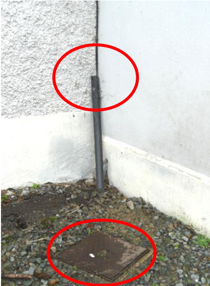
Premises where access box is fitted and duct is fitted on external wall.
