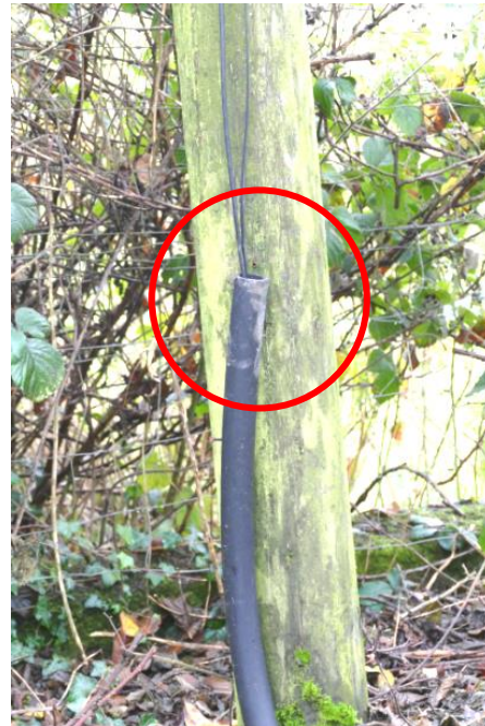
Duct at network touch point. No draw rope present.
