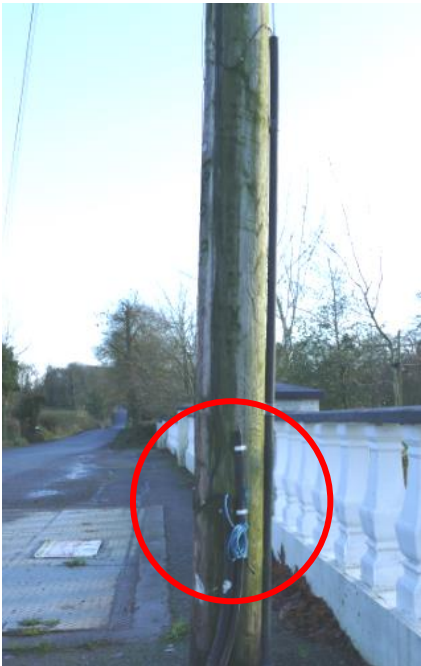
Network touch point with multiple ducts. A draw rope present in one duct.
