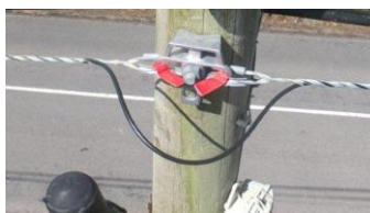
Figure 2 - UPB pole fitting on the opposite side of the pole to the existing copper cable bracket
